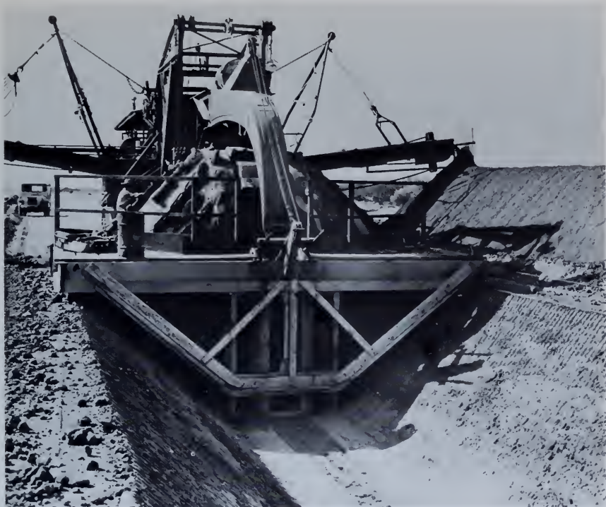
Figure 148. —Excavating a small canal on the Gila project, Arizona. The canal is excavated in a single pass. PX-D-33037.
